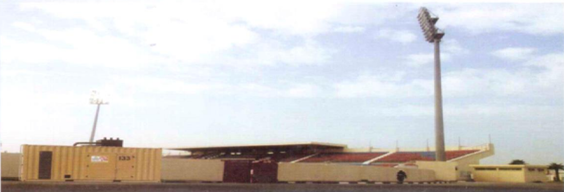
1000 Kva Rental For Stadium
