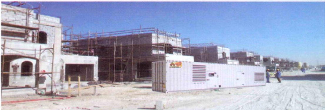
1 MW Rental For Villas Project
