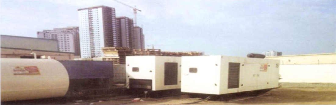
2 Units 500 Kva Rental with Synchronizing System For Water Treatment Plant
