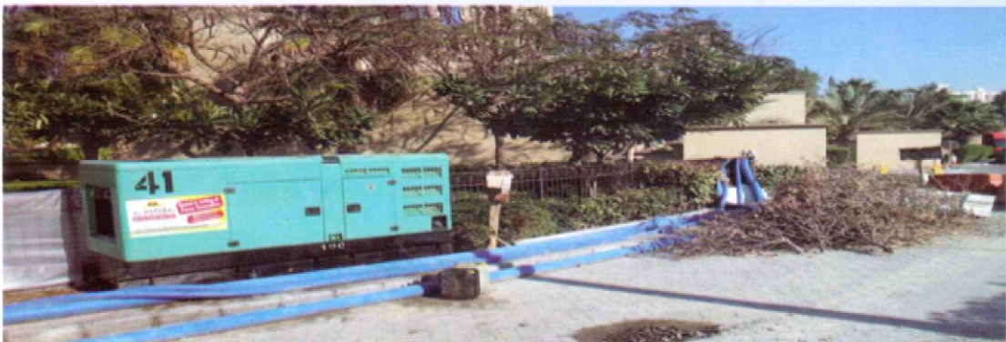
200 Kva Rental For Dewatering
